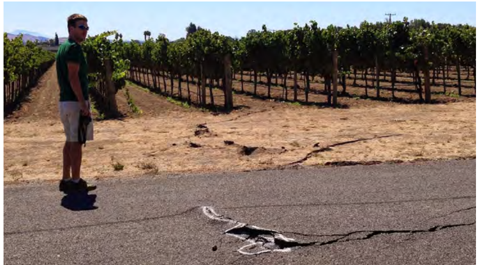
Rupture across South Avenue and adjacent vineyard. Grad student Chad Trexler for scale.
